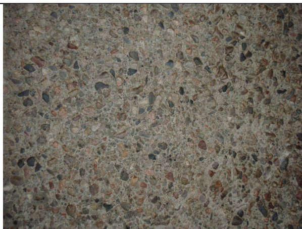
Figur 5.20 Sulfatangrep. (Foto: Norconsult AS)
